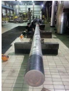
Gambar 5. As Vibro Turbin Compressor
